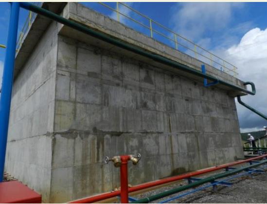
Reator UASB de concreto
